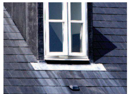
Example of staining when left untreated
