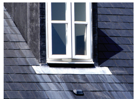
Example of staining when left untreated
